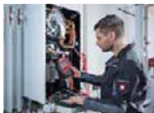
Testing of gas pressure regulators
